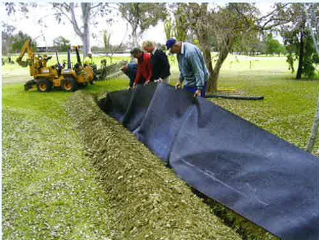
Splitbelt is used as a vertical barrier to prevent tree roots extending under golf greens (Tamworth)
