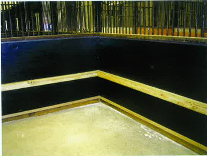
Splitbelt is often used to line stables and minimise injuries to horse’s legs. This installation at Emirates Park is typical of this application.
